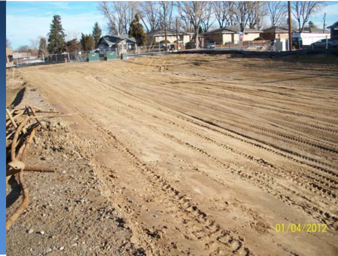
Storm water detention pond in NE corner of site.
