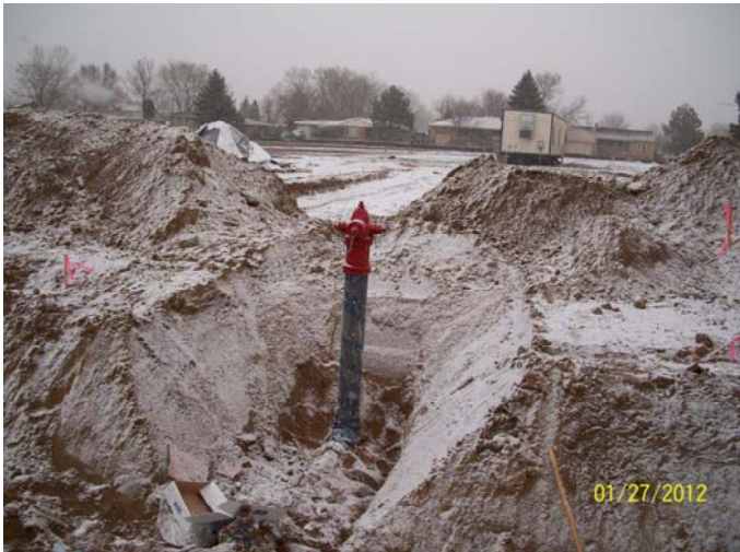
Fire hydrant installed on Vance Street. Waiting for inspection prior to backfill.
